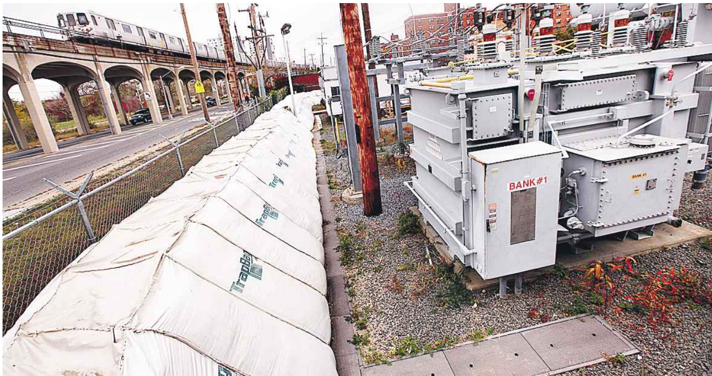
LIPA has placed 6-foot-tall sandbags around the Arverne substation in Far Rockaway to prevent damage from storm flooding.
